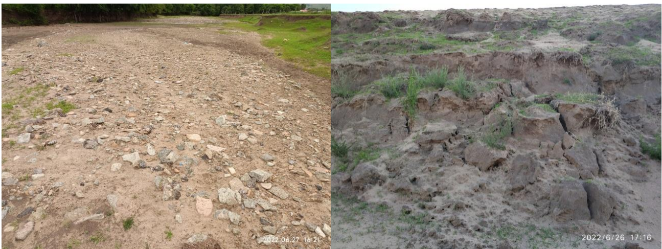
Figure 2: Source of Sediment Accumulation at the Bottom of the Ravine
