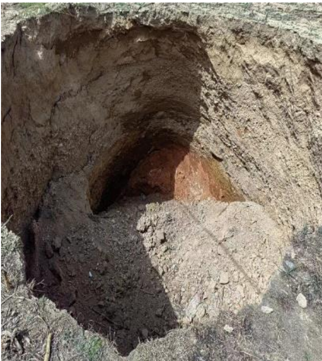
Figure 2: Subsidence Pit Photos
