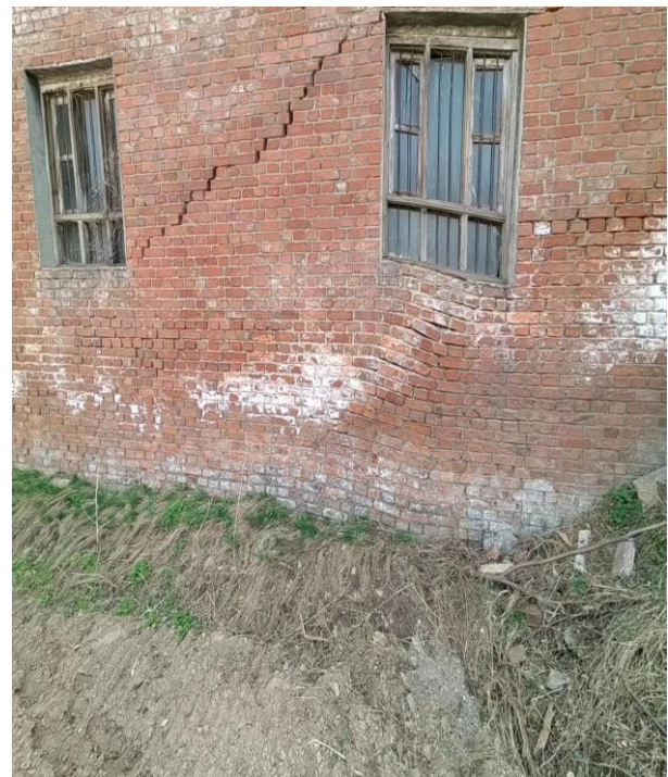
Figure 3: Photos of Cracked Houses
