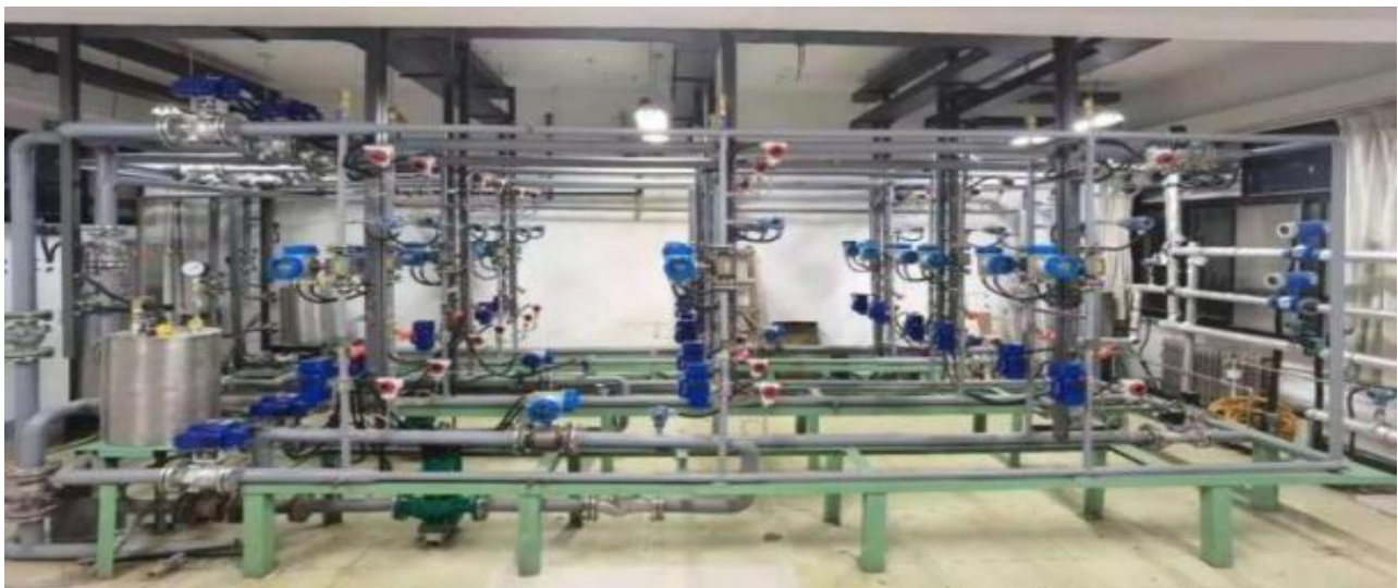
Figure 1: The physical image of the experimental heating-network system
