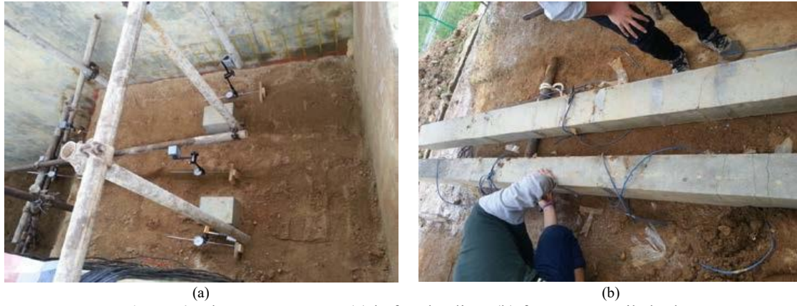
Figure 4: The test processes: (a) before loading; (b) fractures on pile body
