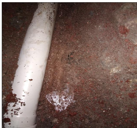
Figure 5: Water near Underground Pipes
