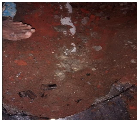
Figure 5: Bricks used instead of Waterproof membrane
