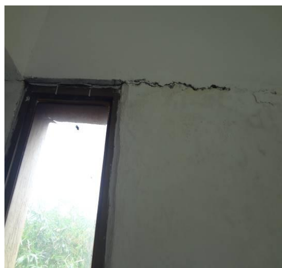
Photograph 11: Beam-wall (Horizontal crack)
