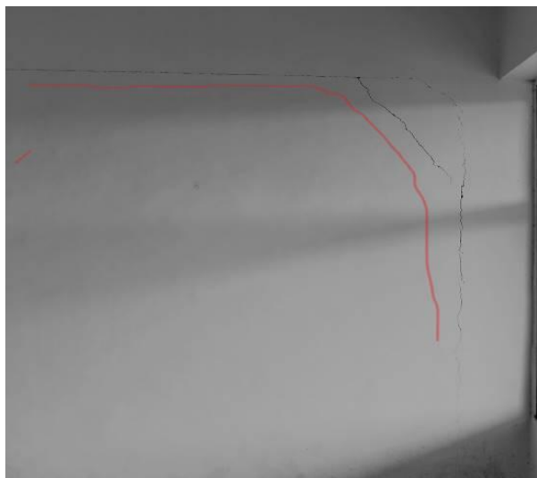
Photograph 7: Joint of column-wall and Beam-wall (Diagonal cracks)
