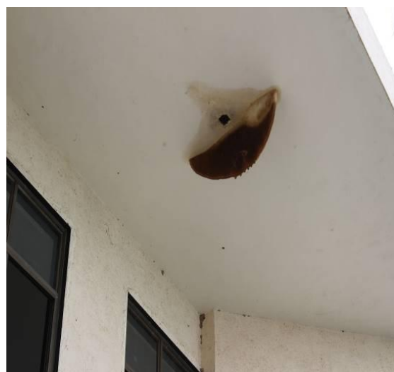
Photograph 12: Lack of maintenance
