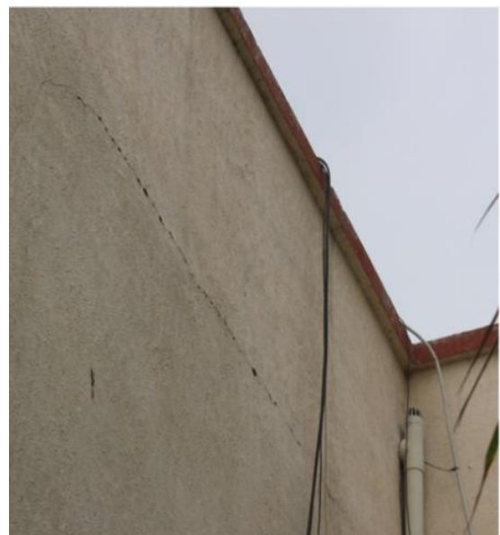
Photograph 6: Horizontal crack due to shrinkage
