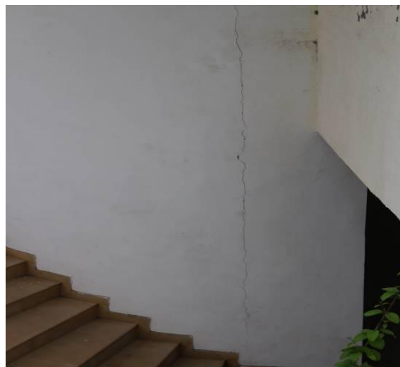
Photograph 10: Beam-wall / Vertical crack (Expansion joint)
