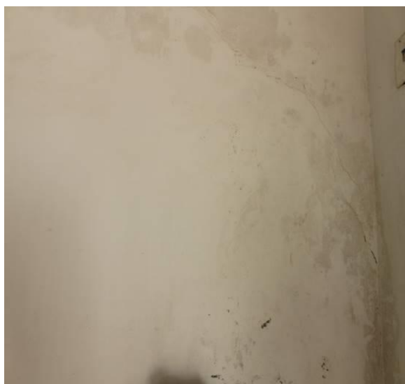
Photograph 8: Near vegetation (Diagonal cracks)
