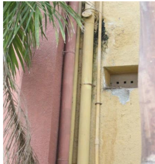
Photograph 5: - Improper/poor drainage pipe
