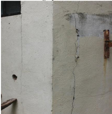
Photograph 2: Vertical crack (Wide crack) Due to Thermal stress
