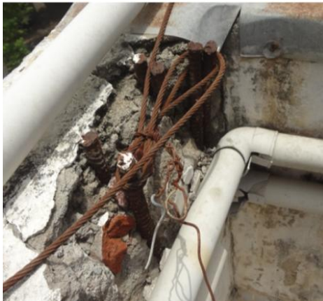
Photograph 3: Open reinforcement and Environmental Effect
