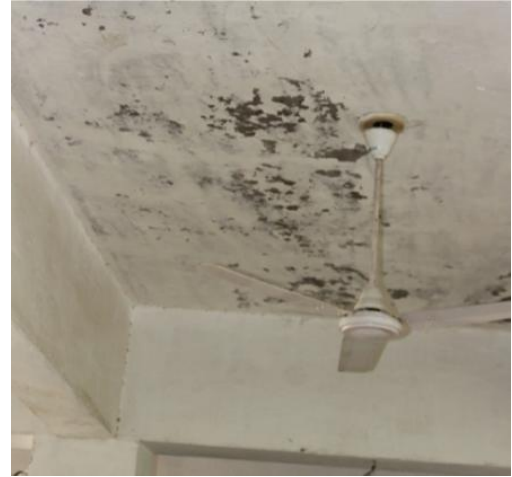
Photograph 4: Leakage and Dampness
