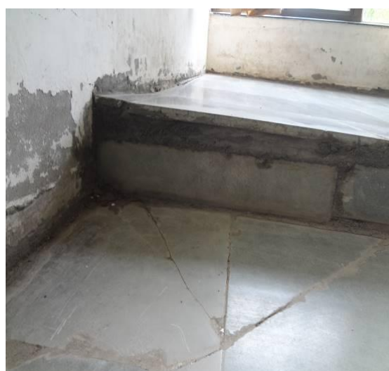
Photograph 9: Flooring/ Improper leveling
